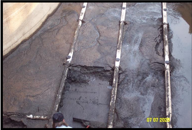
Beginning July 6 th , contractors were on site to remove grit from the aeration tank & digester.
