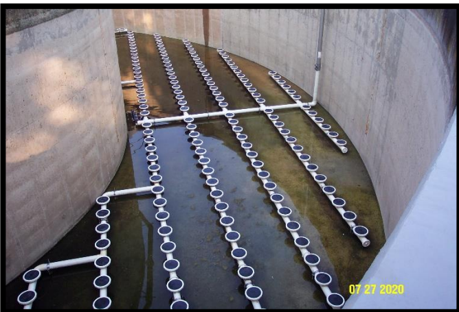
WWTP & WTP staff worked to complete the installation of 490 total new Sanitaire diffusers.
