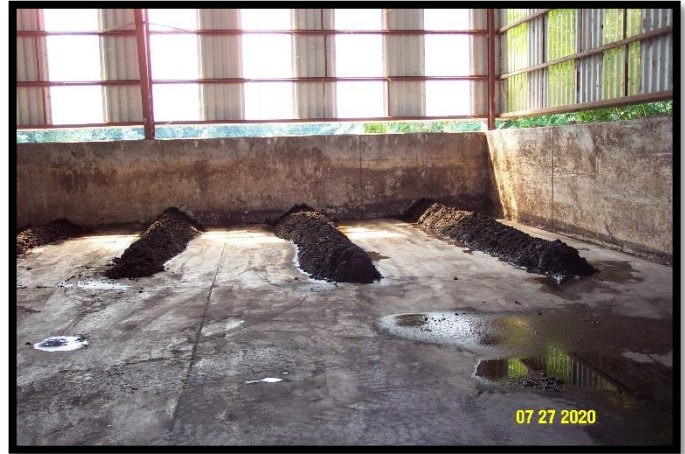
Grit removed from aeration tank dewatering in the bio solids building, organized into windrows.
