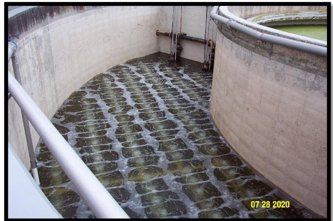
Completed aeration tank cleanout project with the blower on and the diffusers in operation.
